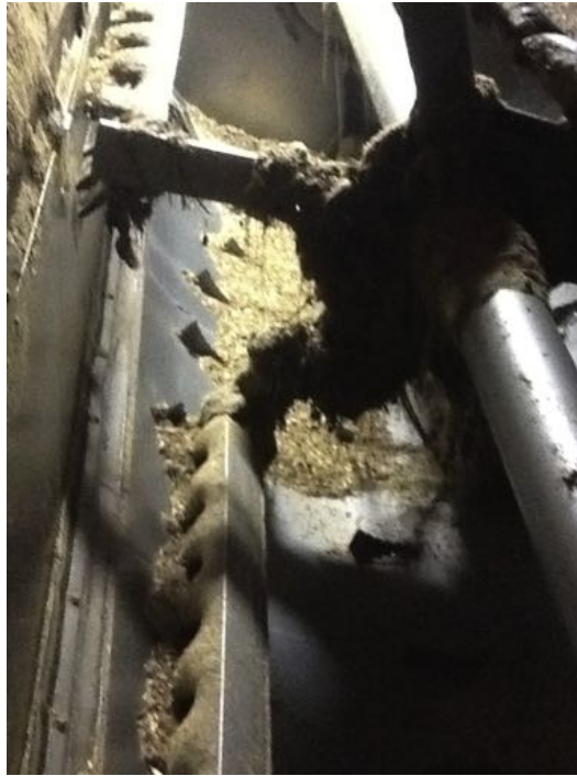
Fig. 11. TMR under the front part of the mixer rail indicating a bent or worn rail.
